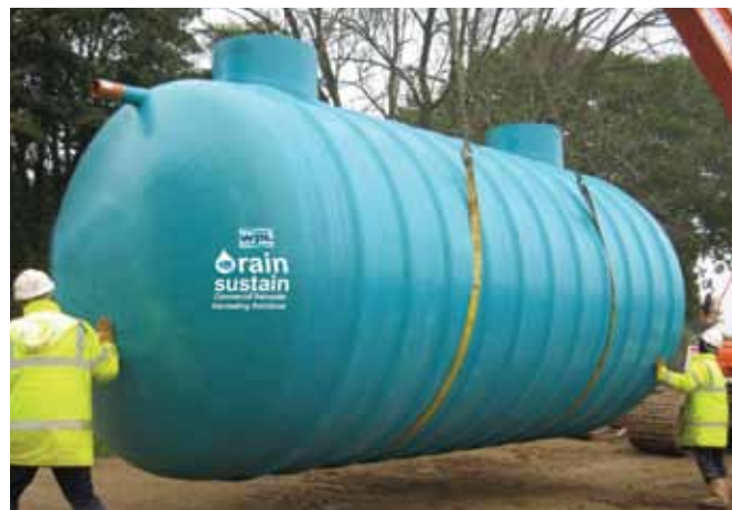
Figure 5 → Examples of underground storage tanks
