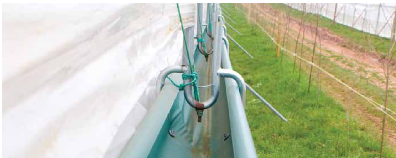
Good guttering is vital to capture rainwater
