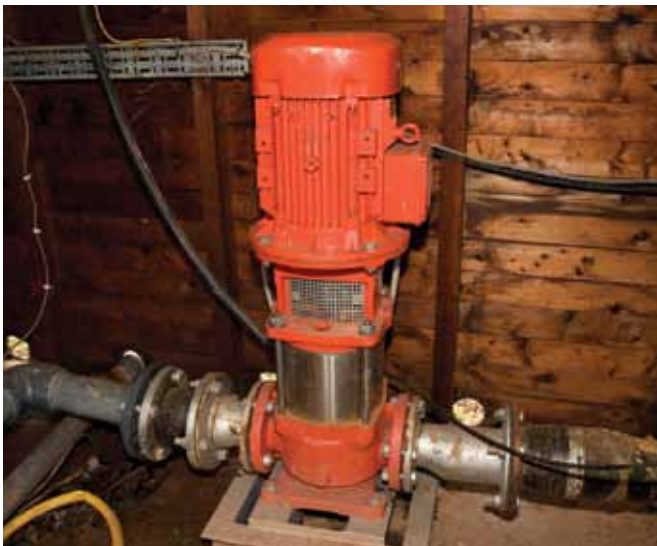
Pumps are needed to ensure the right pressure for the use of water
