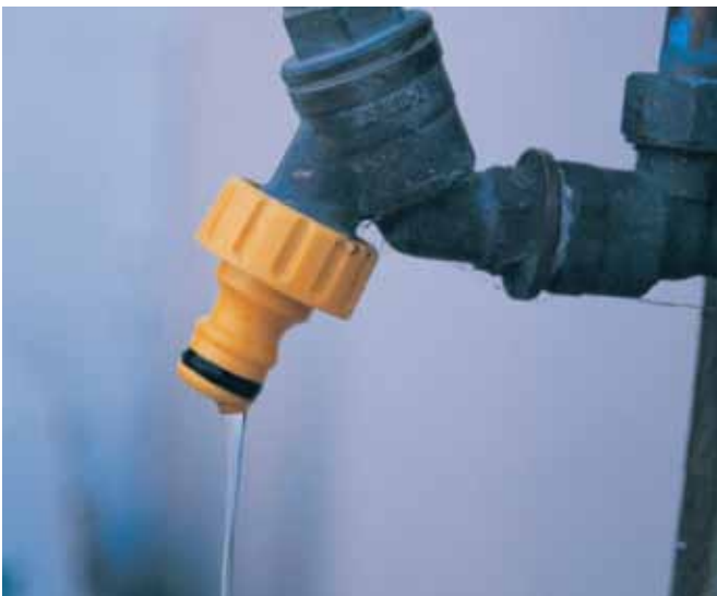
Before considering new sources of water supply identify where you may have leaks first
